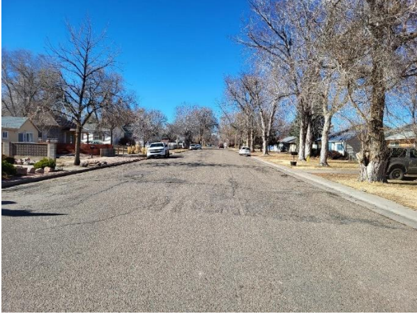
3 3rd St- example of typical city pavement condition
