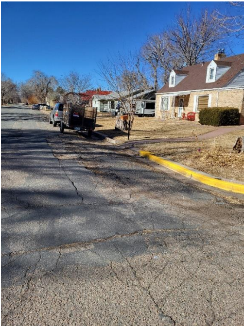
4 4th St- localized severe pavement damage.
