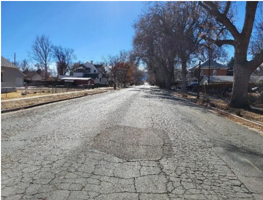
6 Alligator cracking at Robinson and 4th St.
