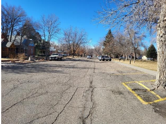
8 Poor pavement condition near the park
