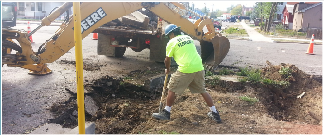
Florence Public Works department installing an ADA ramp in a busy intersection. New sidewalks (bottom left) and curb cuts installed by the PWD.
